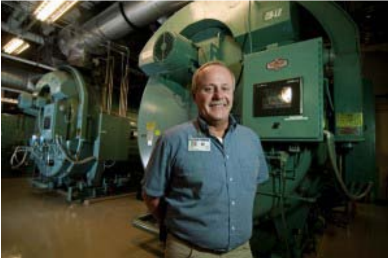
Steve Matherly, an engineer at the Legacy Salmon Creek Medical Center in Vancouver, Wash., stands in front of a pair of natural gas-powered water heaters used to warm recirculated air. Matherly was a member of the team that participated in a study aiming to help decrease energy use in hospitals. (Photo by Sam Tenney/DJC)
